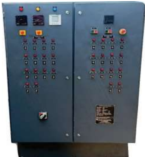
400 kW RL Load Bank
