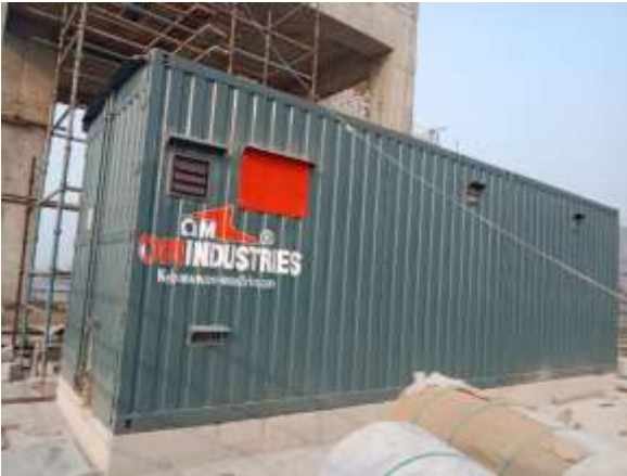
2000 kW RL Load Bank, NTT, DC02, Dighe, Navi Mumbai
