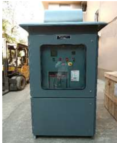
400 kW Load Bank, NTT, Dighe, Navi Mumbai
