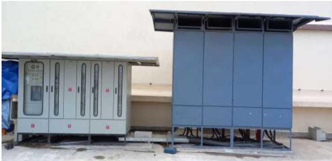
2200 kW Resistive Load Bank NTT, DC08, Chandivali, Mumbai
