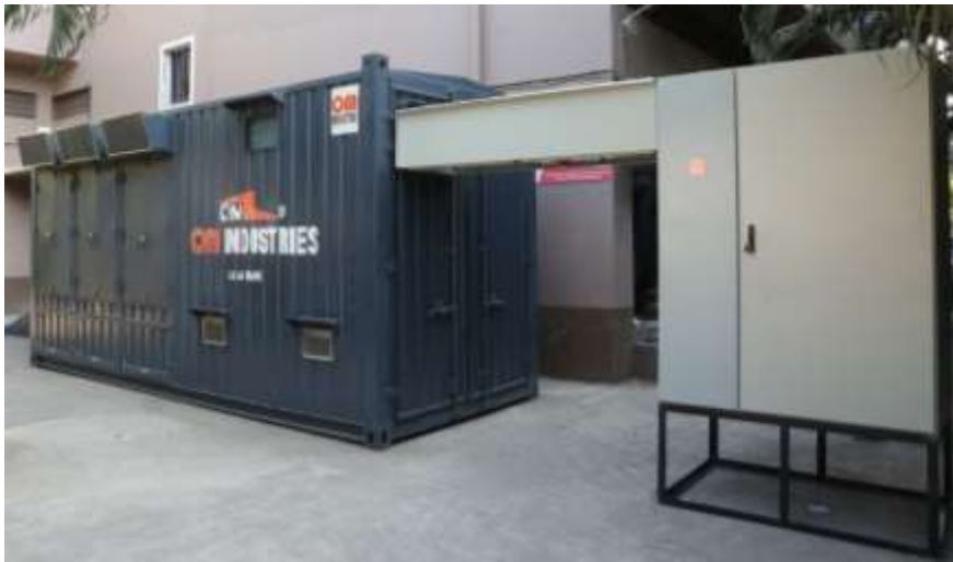
2000 kW RL Load Bank, NTT, DC01, Dighe, Navi Mumbai
